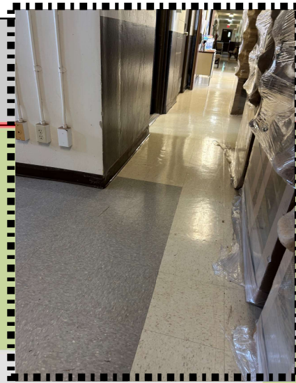
EXISTING FLOORING CONDITIONS: PORTIONS OF THE LOBBY (GREY VINYL TILE) AND HALLWAY (BEIGE VINYL TILE)
